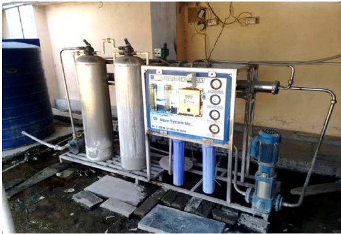
Fig.3 RO Plant use to purified the ground water for machine
