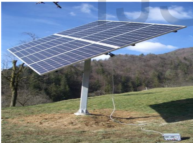
Fig 2. Photovoltaic Tracking System
