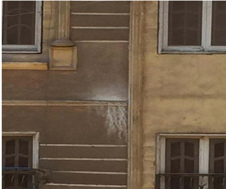
Figure 4. Efflorescence of walls in residential building, Cairo, Egypt.
