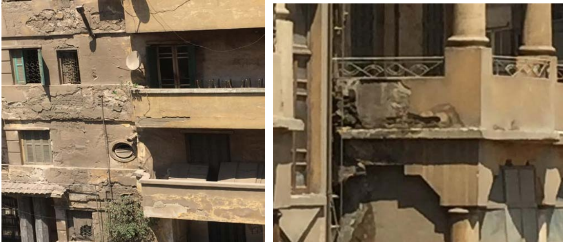
Figure 1. Weathering of old buildings at Zaitoun area, Cairo, Egypt.
