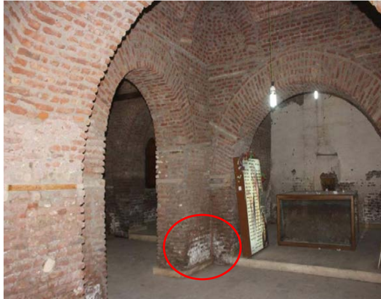
Figure 3 Salt attack for masonry wall at St. Demiana Church, Belqas Dakahlia, Egypt
