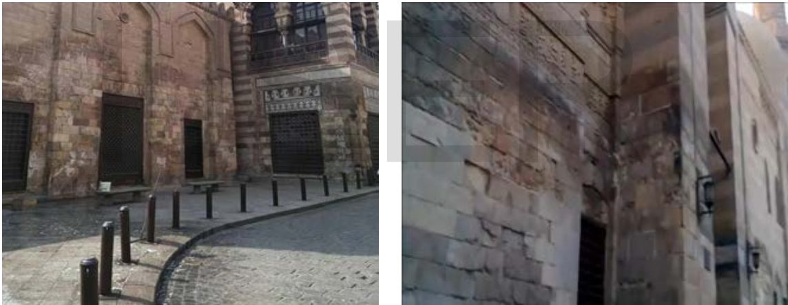
Figure 2. Salt weathering of stone frontage of historic Building at Moez St. Old Cairo, Egypt.
