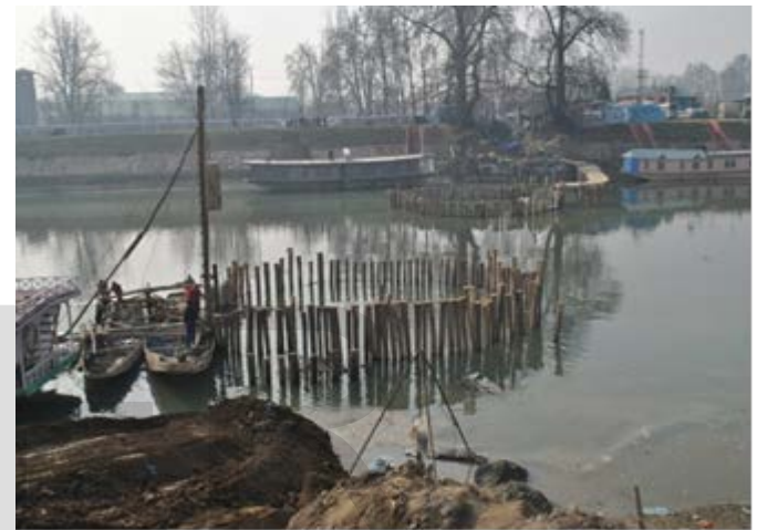
(Fig. 1 First stage of well foundation. On going project near convent school in Kashmir)
