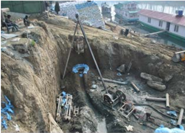
Fig. 4 .A hammer is inserting the casing in the bore hole by winch crab. This is the first stage of the pile foundation. The method used for the construction of the pile here is direct mud circulation method.
